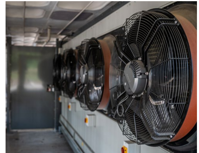
At Wolfson College Oxford, external air source heat pump installations were rarely found to cause problems with noise, appearance, or cold air discharge when sensibly located and properly detailed.
