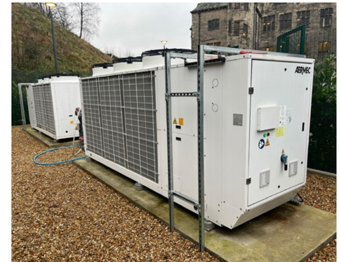
Air source heat pumps can be successfully integrated into historic settings when thoughtfully sited and detailed, without compromising the character of the building.
