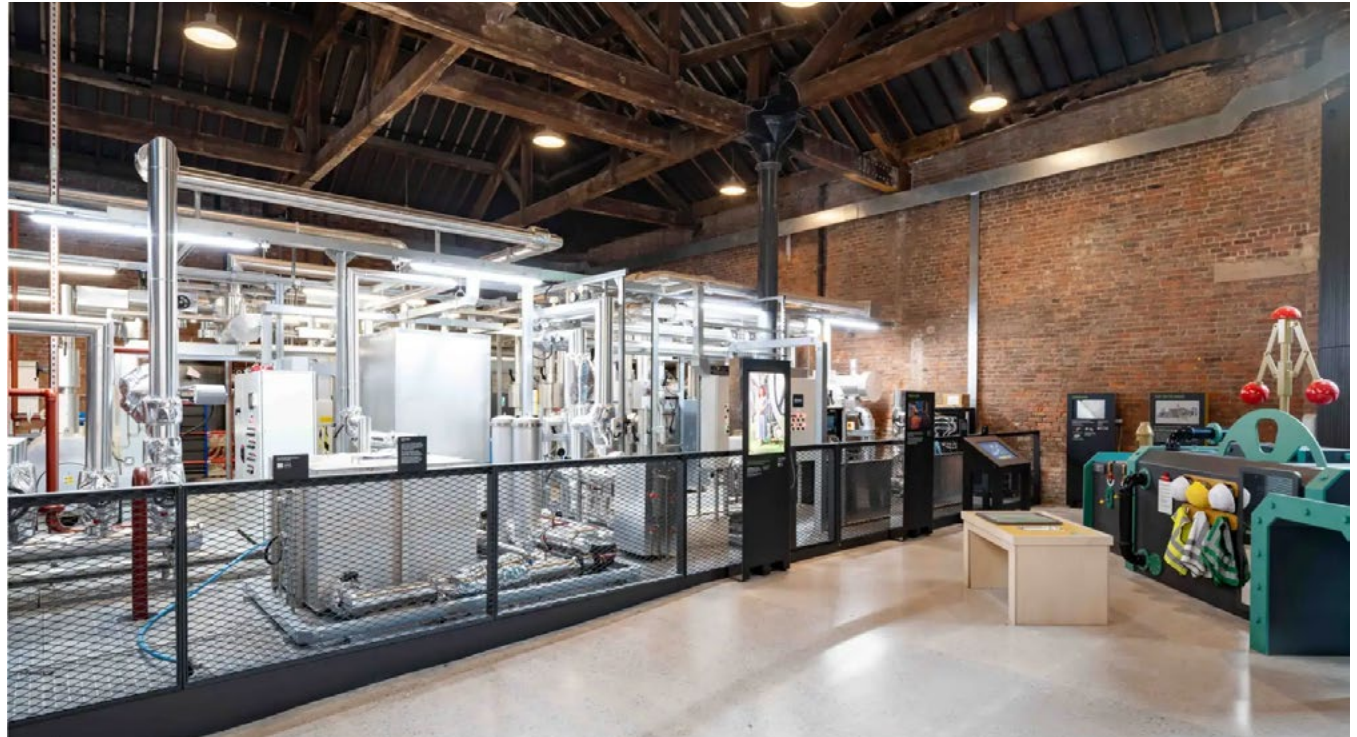
The MEP plant room is proudly on display at Power Hall as part of explaining and showing and understanding how machines and systems operate.
