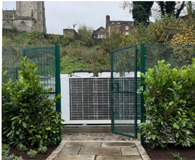
Air source heat pumps can be successfully integrated into historic settings when thoughtfully sited and detailed, without compromising the character of the building.
